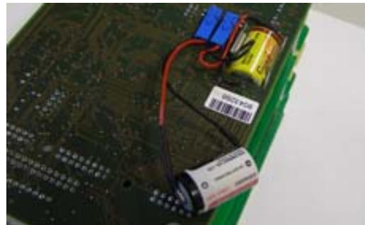
Parallel arranged batteries
