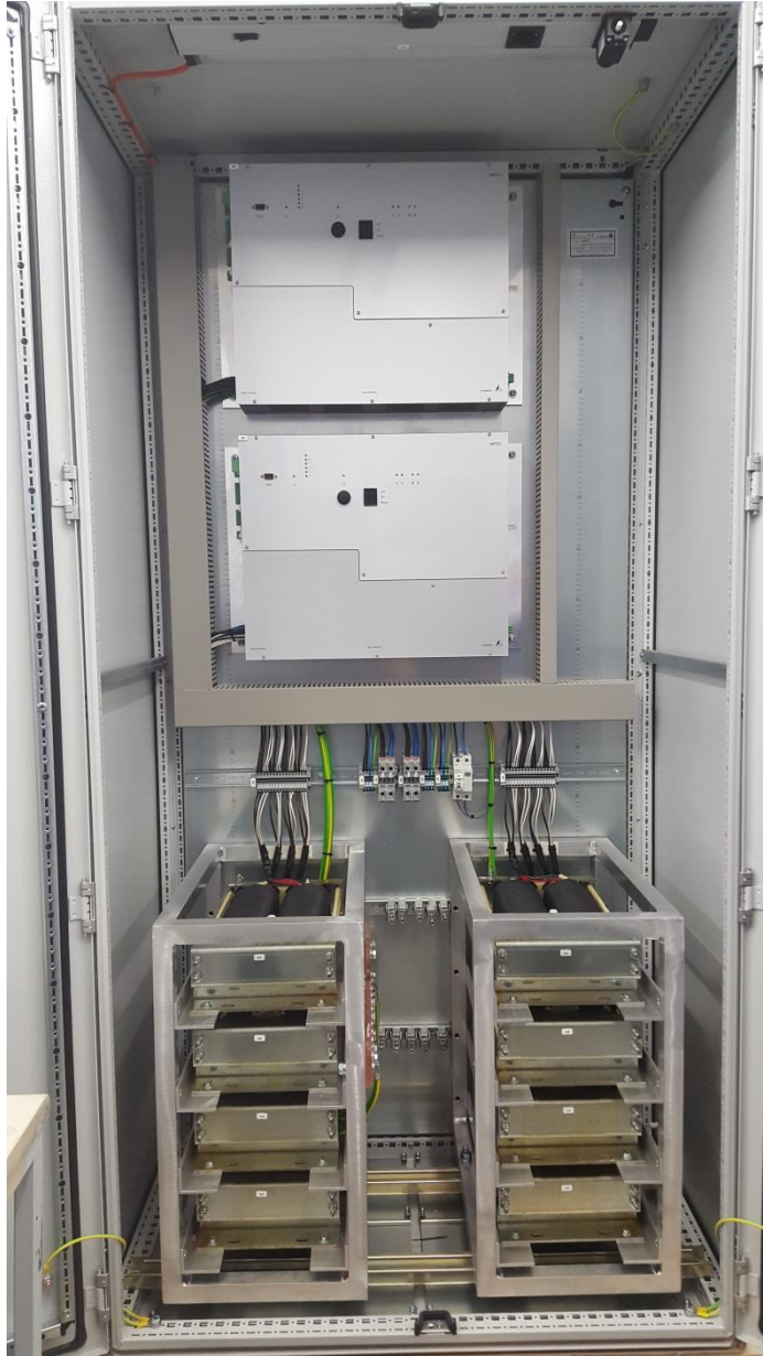
Figure 145: The structure of a dual HPCI – for two REG-DP/ REG-DPA or two P-coils
